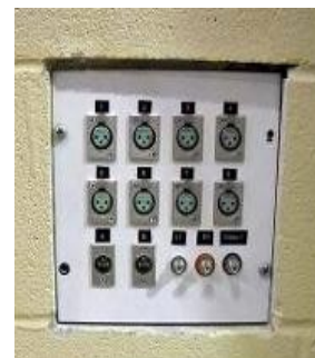
Full Audio Visual Hookups On Each Wall. Fellowship Hall Has 2 750 Watt Self Powered Speakers connected to a 16 channel
